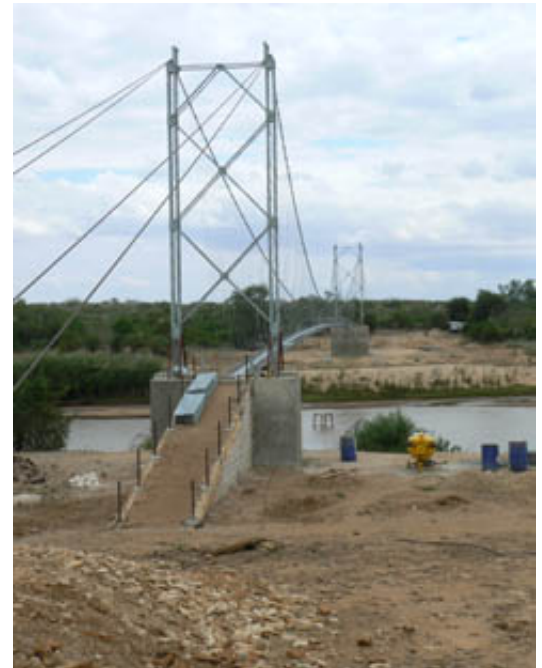
With a span of 112m, the structure is considerably longer than others built by the charity
